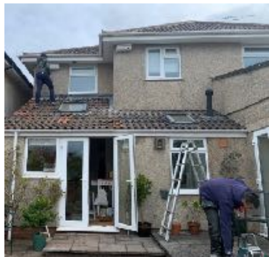
Boxes going up ready for the swifts. Hopefully in 2025 more swifts will return to the colony in Wrigton Lane.
